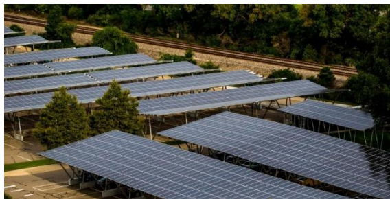
Solar canopy above surface parking lot.
