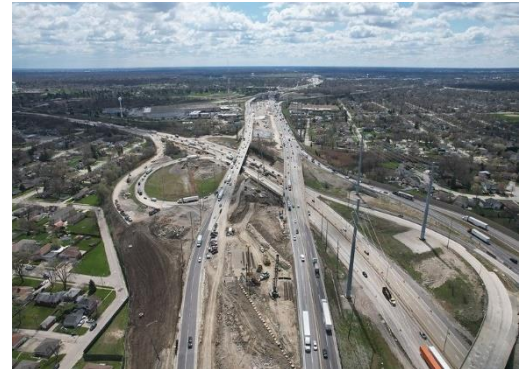
I-290/I-88 Interchange Project at I-294. Progress at I-290 facing south near Berkeley.
