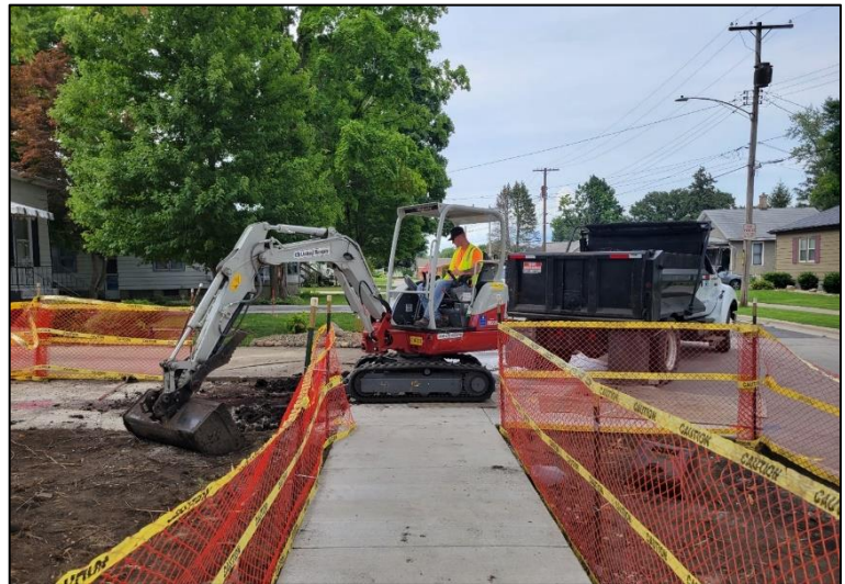
Residential cleanup at a Superfund site in the City of La Salle
