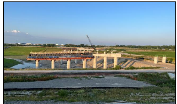
Bridge piers are constructed along the Jane Addams Memorial Tollway (I-90) as part of the I-490/I-90 interchange near Des Plaines
