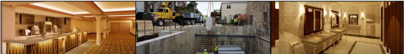
New concession space, installation of an air conditioning unit, and a new restroom at the Egyptian Theatre
