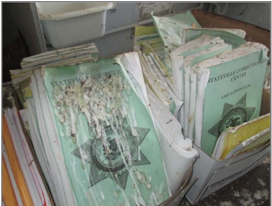
Documents have been destroyed due to birds infiltrating a few rooms. Department of Corrections - Stateville Correctional Center - Joliet
