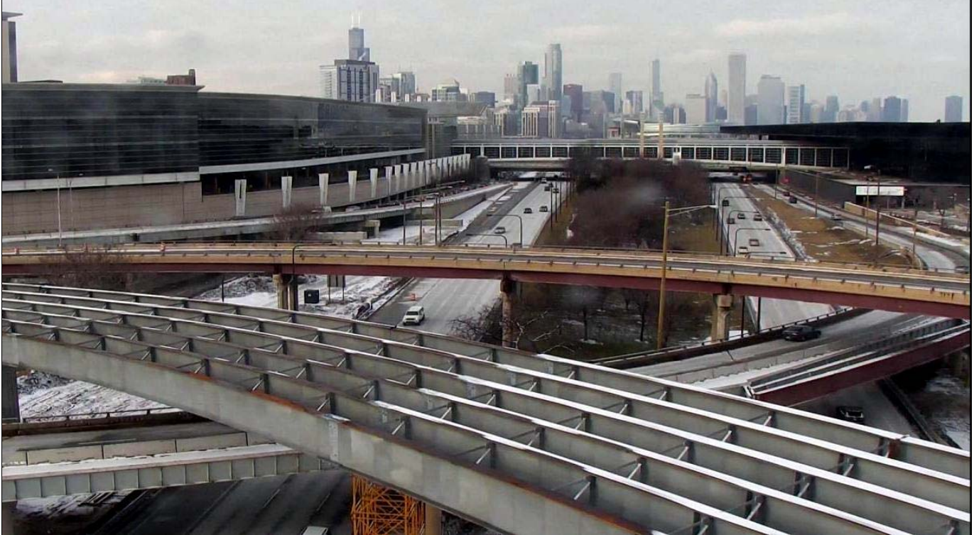
New bridge under construction connecting northbound Lake Shore Drive to outbound I-55.
