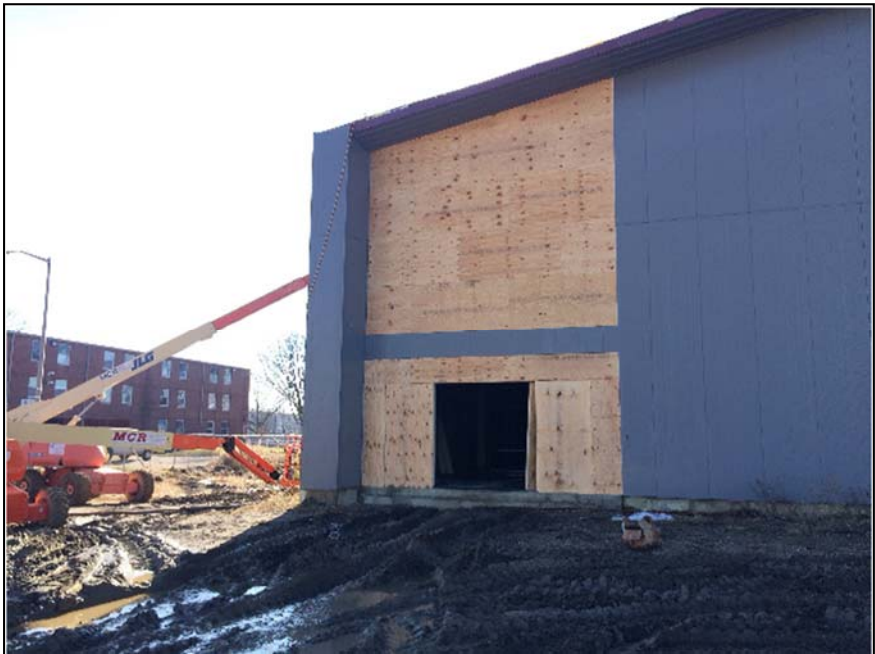
Temporary plywood walls were installed to keep winter weather out of the partially completed gymnasium. Department of Military Affairs - Lincoln's ChalleNGe - Rantoul
