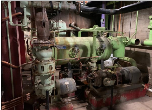
Boiler to be replaced at Elgin Mental Health Center
