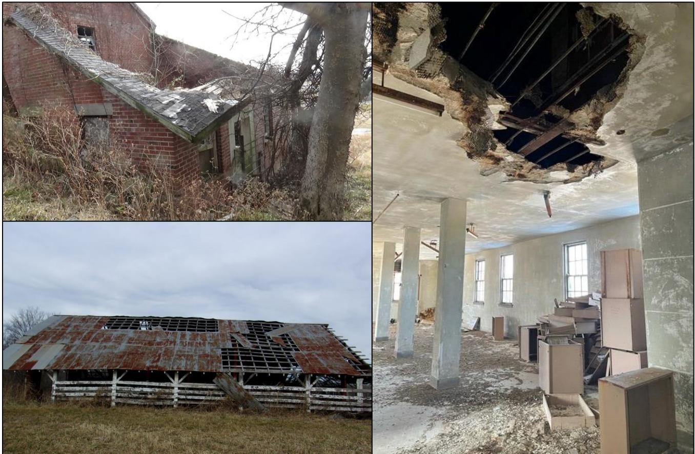
Visibly deteriorated structures slated for demolition at DOC facilities. Top: Loafing Barn at Menard Correctional Center; Bottom: East Barn at Vienna Correctional Center; Right: Dixon Correctional Center Cold Storage Building
