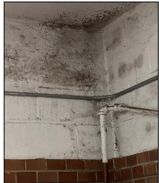
Mold in the Logan Correctional Center gym is being remediated by CDB.
