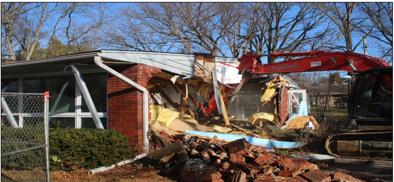
Demolition of flood prone structures as part of the flood mitigation buyout program
