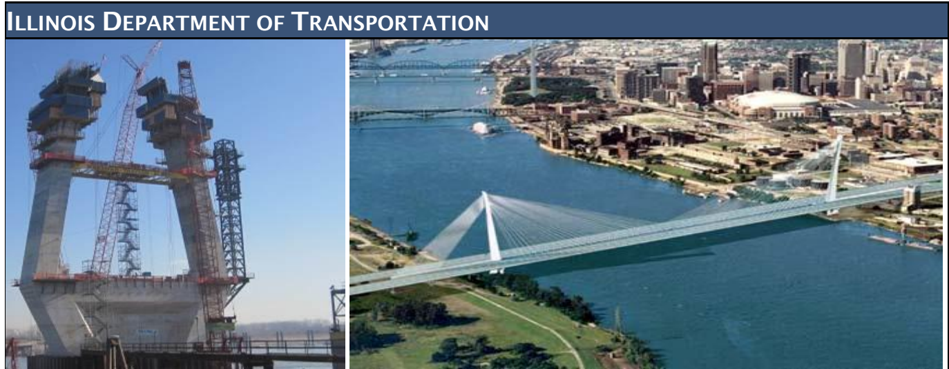
The New Mississippi River Bridge Project, a joint project with the Missouri Department of Transportation.
